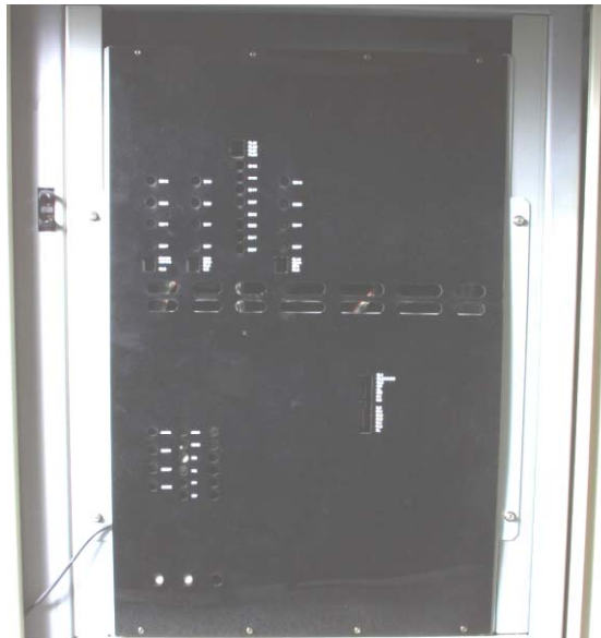
Fig. 4.6 Control panel R2
